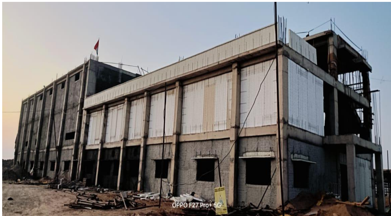
NTPC Renewal Energy Ltd Solar Farm Project Khavda, Gujarat
