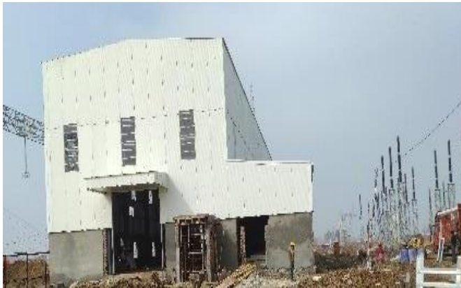
PEB GIS Building, L&T, Meerut, UP
