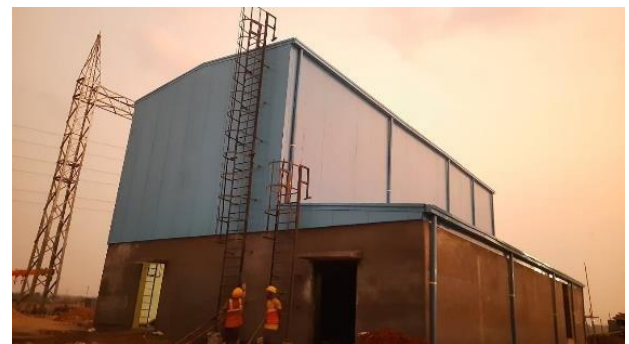
PEB GIS Building, TOSHIBA Godishahi, Odisha
