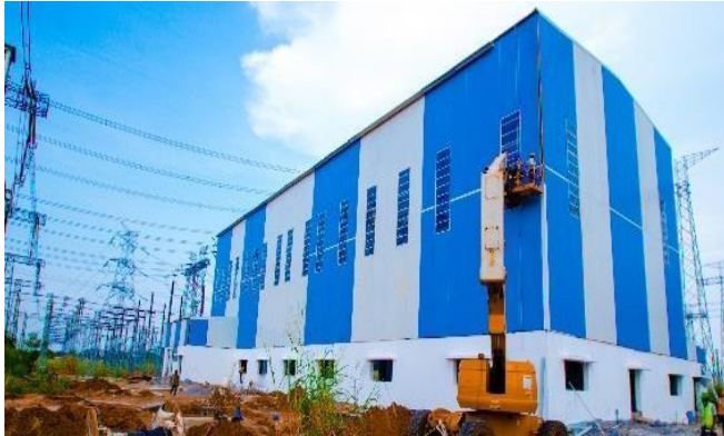
PEB GIS Building, GE T&D, Phagi, Rajasthan
